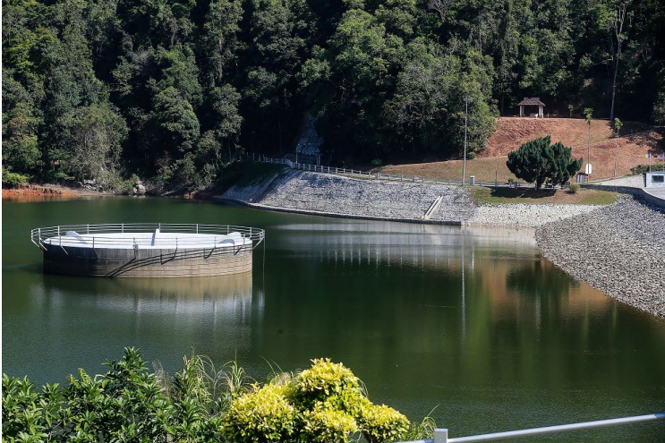
A view of the Air Itam dam March 12, 2021. — Picture by Sayuti Zainudin
