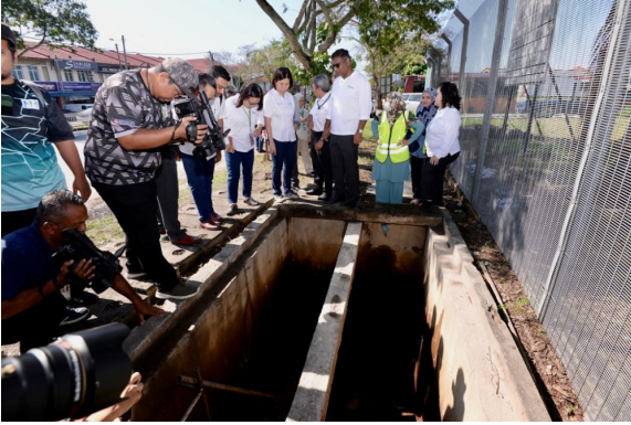
Penang Water Supply Corporation chief executive officer K. Pathmanathan and his team check on another valve at the Sungai Dua Water Treatment Plant that needs to be replaced, December 13, 2023. — Picture by Opalyn Mok
