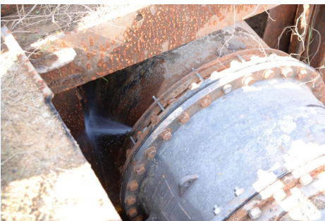
One of the valves at the Sungai Dua Water Treatment Plant that needs to be replaced, December 13, 2023. — Picture by Opalyn Mok
