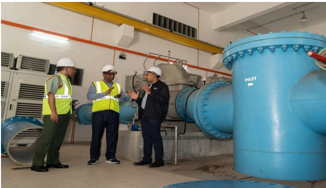
APRIL 2025 SWSI: "GREEN LIGHT" FOR 23 WATER WORKS PROJECTS © PBAPP 2025 3 projects to upgrade treated water re-pumping operations at the Bukit Dumbar Reservoir and Pumping Station Complex
