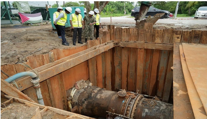
APRIL 2025 SWSI: "GREEN LIGHT" FOR 23 WATER WORKS PROJECTS © PBAPP 2025 Replacement of a faulty 1.2m valve at a pipeline in Jalan Pengkalan Tambang, near the Sungai Dua WTP in SPU.
