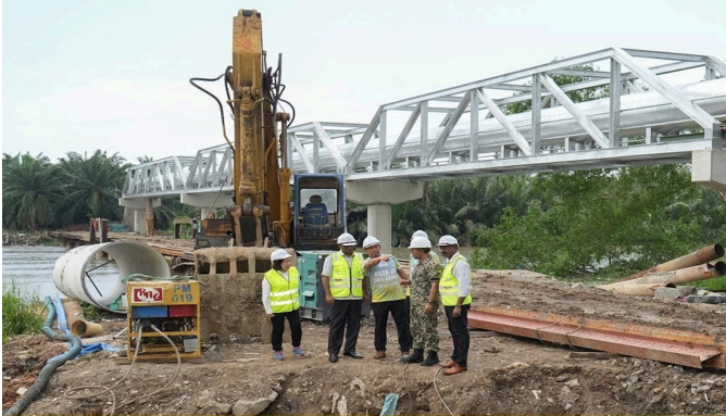
APRIL 2025 SWSI: "GREEN LIGHT" FOR 23 WATER WORKS PROJECTS © PBAPP 2025 Final connection works for the 1.35m Sungai Perai River Crossing Pipeline in Seberang Perai Tengah.
