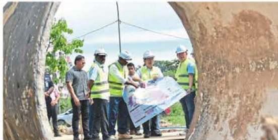
Chow (second from right) checking the progress of work on the pipeline diverted across the Ampang Jajar bridge on the river surface of Sungai Perai in Butteworth. — Courtesy of Buletin Mutiara
