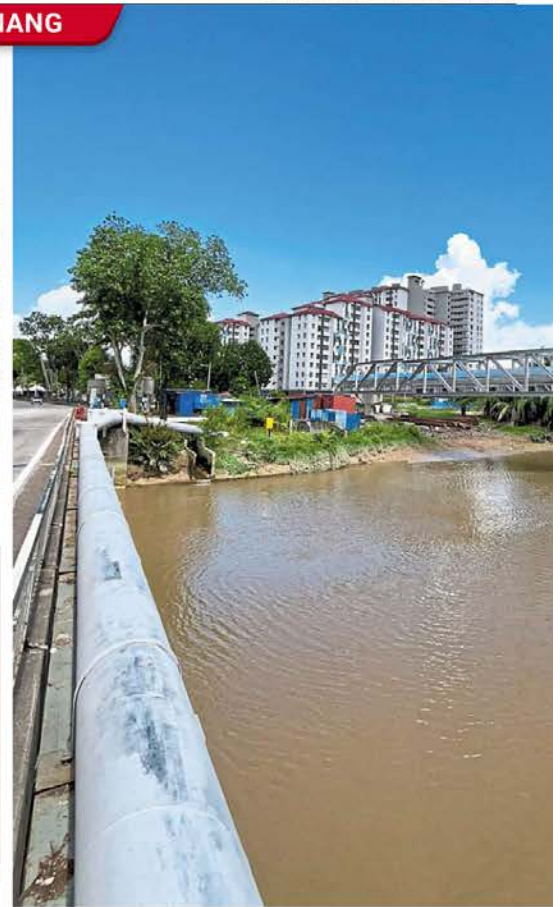
Workers dismantling the temporary platform for the construction of the RM8.7mil Sungai Perai River-Crossing Pipeline (SP-RCP) in Mak Mandin, Butterworth. — ZHAFARAN NASIB/The Star
