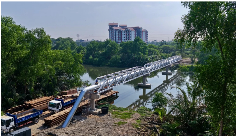
Kerja penyambungan akhir paip menyeberangi Sungai Prai (SP-RCP) siap pada 26.4.2026. The final connection works for the 3rd Sungai Prai River Crossing Pipeline (SP-RCP) was completed on 26.4.2026. © PBAPP 2026
